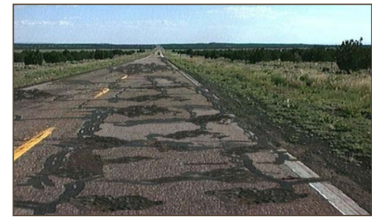
LOS F: This pavement is impassable.
